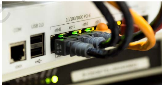
Figure 10.12: Cables connected to a network switch
